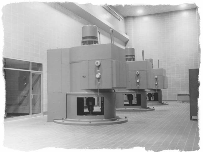
New pumps at North Point Station, 1964.
